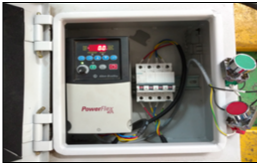
Fig. 7. Variable Frequency Drive (VFD).
