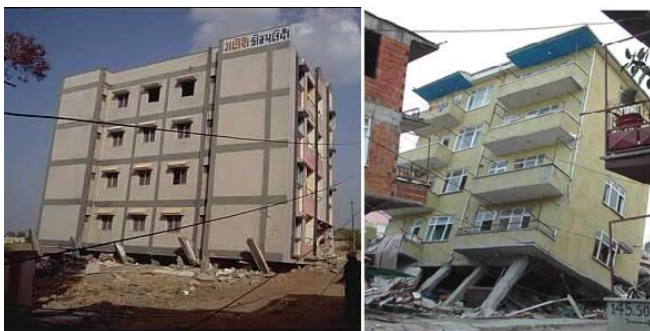
Figure 1. Soft and weak storey failure due to large lateral displacement
