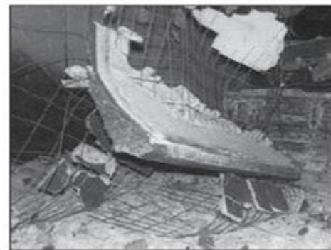
Surface cracking after Structural failure subjected to high temperatures.
