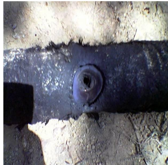
Figure 5. Cable Fault In A 132kv PILC Cable
