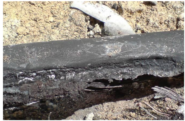
Figure 4. Vaporized Core After Cable Fault, 132kv XLPE
