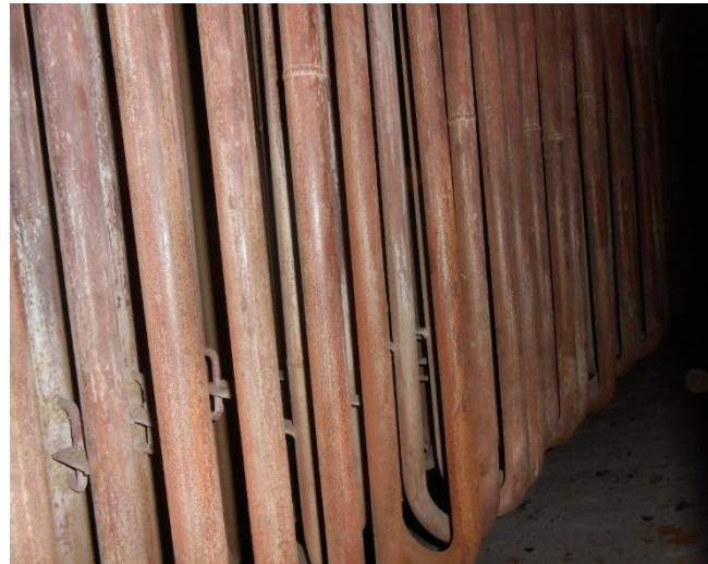
Figure: 1 Actual Photograph of Superheater inside Boiler
