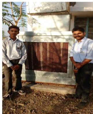
Figure: 3.3.3. Evaporative Cooler
