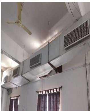
Figure: 3.3.2. Duct System in Seminar Hall
