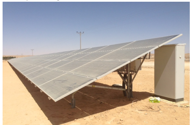
Figure 1. Dust on Solar Panel.
