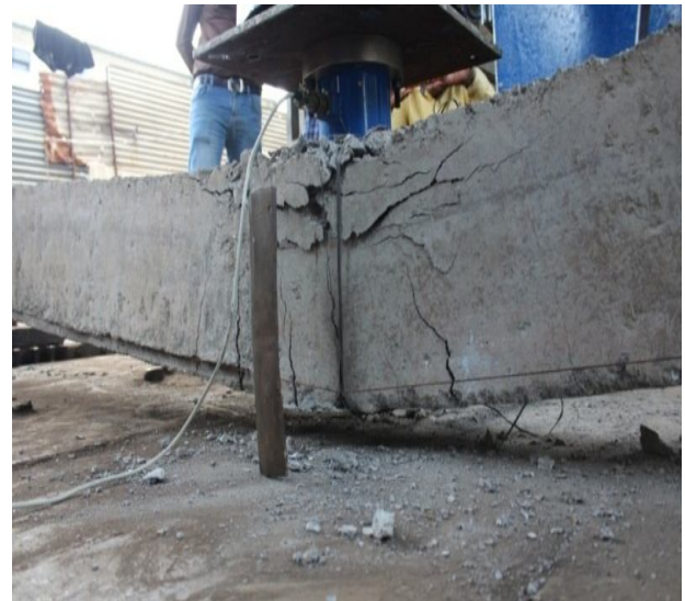
Photo No. 3.5: Beam failure at maximum load.
