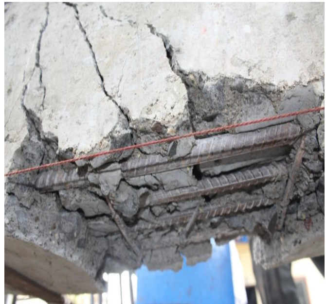
Photo No. 3.3: Reinforcement after failure of beam.
