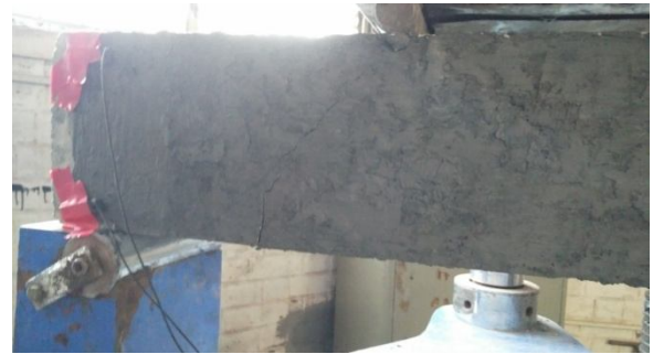
Figure 10. Crack on surface of B3
