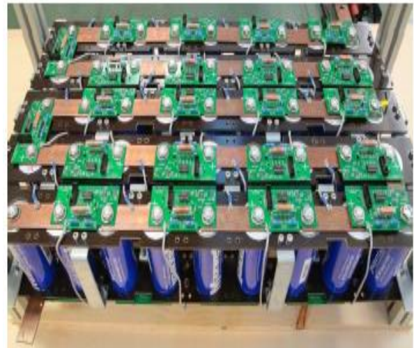
Fig.7: 45 SC stack with buck-boost converter [4].
