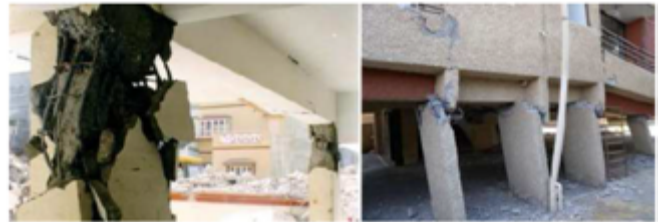
Fig 1.1: Columns that are damaged in soft storey during earthquake
