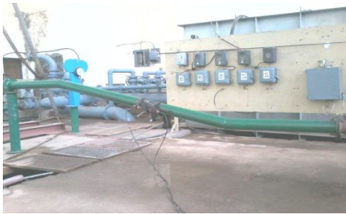
Fig. 3: Ultrasonic flow meter installed at 6° sloped pipe
