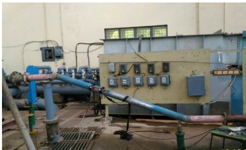
Fig. 4: Ultrasonic flow meter installed at 24° sloped pipe
