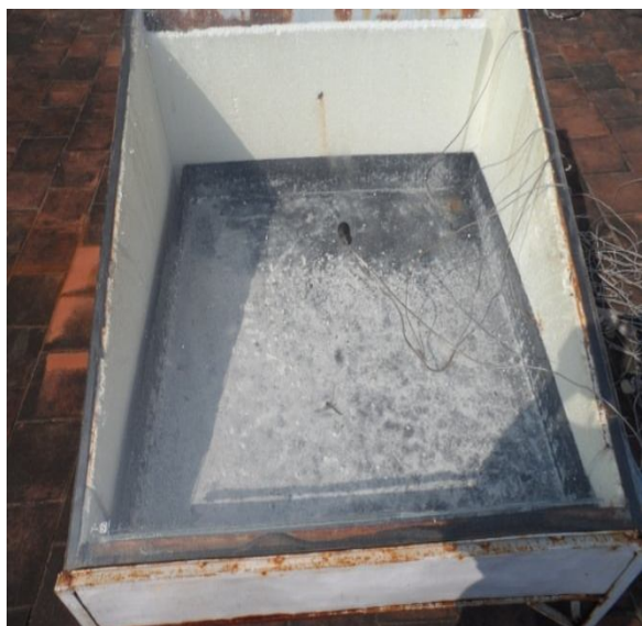
Fig. 11 Photographic view of after removing the scale on Galvanised Iron basin material
