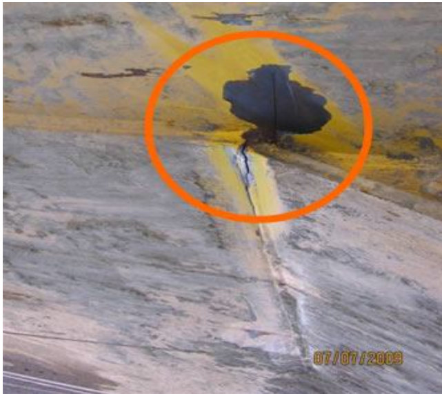
Fig: Fatigue Failure of Hydraulic Scissor lift
