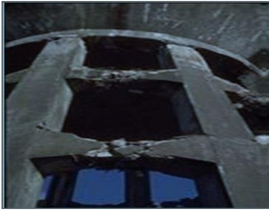
Fig 1. 1:Bending Shear Failure in beam
