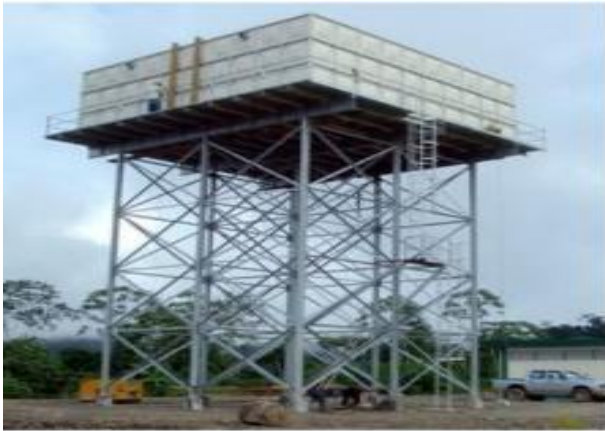
Fig 1: Elevated water storage tanks (ESR)
