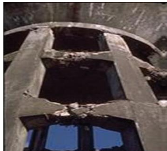
Fig-2: Bending-Shear Failure in Beam
