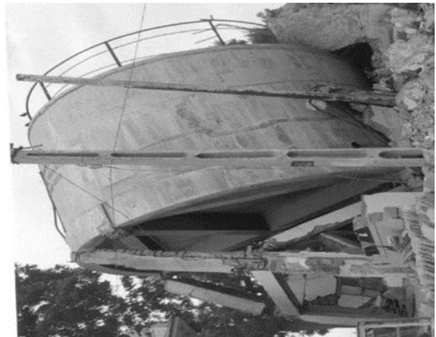
Fig-1: Collapsed Slender and Weak Framed Staging of Water Tanks in Bhuj Earthquake
