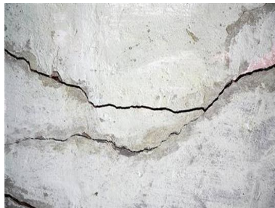
Fig. 1 Cracking of concrete
