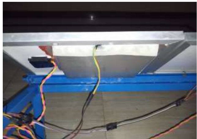
Figure 2 the solar Panel with aluminium chamber containing the PCM.
